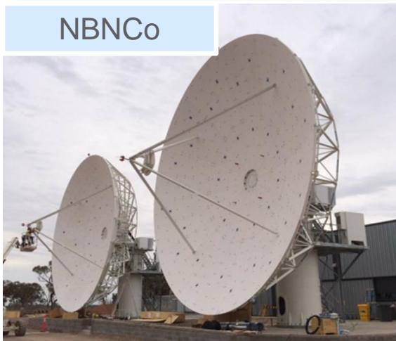
First gateway installation
